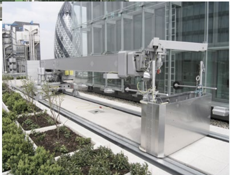
Type 6.1 BMU with a double telescopic jib on a track system integrated in a green roof system.
